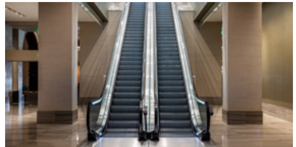
1ST FLOOR ESCALATOR
